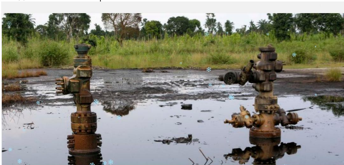
Fig. 2. The plant area contaminated with oil waste.
